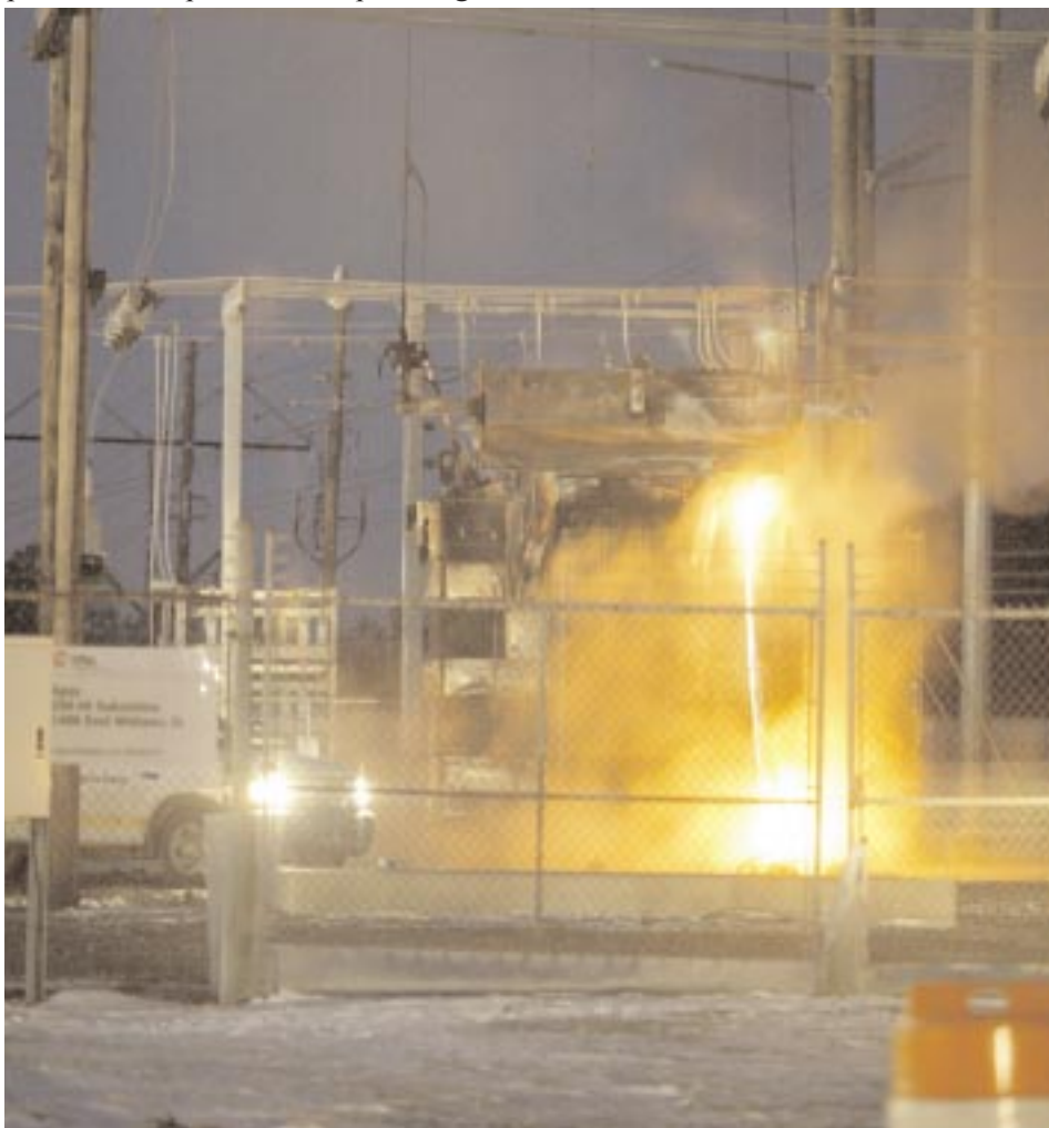
Figure 1-8. A transformer fire at an electric power substation in Apex, North Carolina. Lightning strikes at substations can disrupt electrical service to an urban community for variable durations. (AP Wide World Photos)
