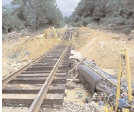
Figure 3-DOT-8. Track washed out by flood waters from Hurricane Alberto.
