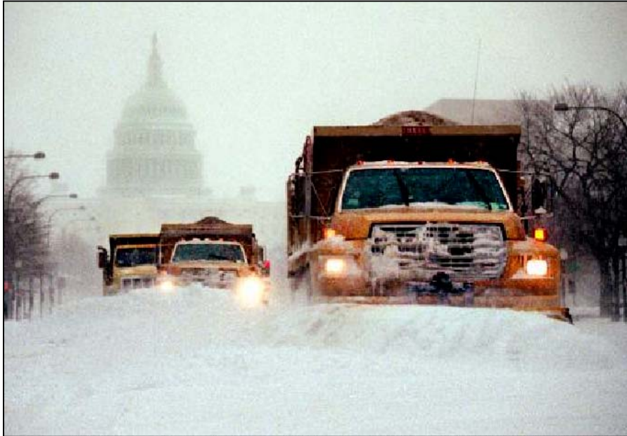
Snow removal is a major road maintenance cost for many states. Better WIST implementation can help reduce these costs, while improving service and safety for highway users. Copyright AP Wide World Photos.
