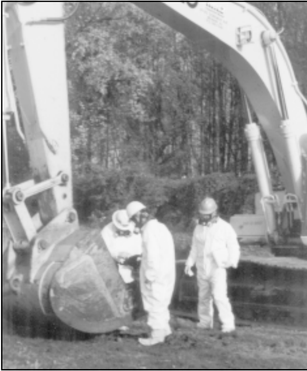
Workers excavate unidentified buried steel drums and heavy-metal-contaminated soil at the Warminster, Pennsylvania site.
