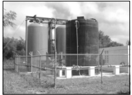
The granular activated carbon system shown here removes organic pollutants from groundwater at Guam.
