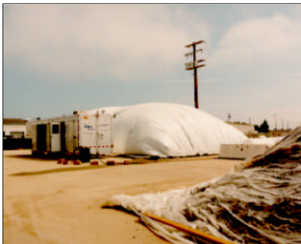
Figure 2. Soil pile is covered by a membrane and ducts are connected to the HAVE system located in the trailer.
