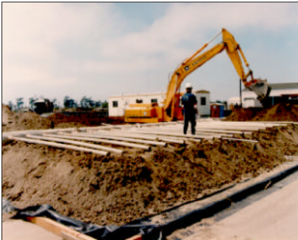
Figure 1. Soil is built into a pile containing ducts for hot air distribution and vapor extraction.
