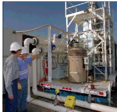
Figure 1. Photolytic destruction system adsorber tank.
