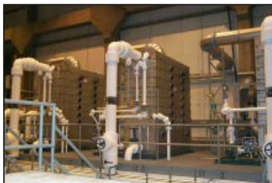
Air Stripping System at NIROP Fridley
