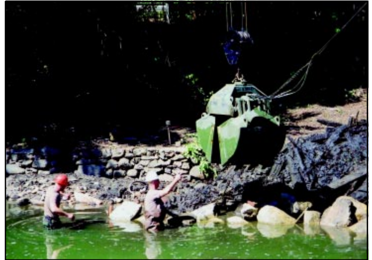
Members of the U.S. Army Reserves removed the Billington Street Dam in Massachusetts as part of the Pilgrim Trail Restoration Partnership Project.
