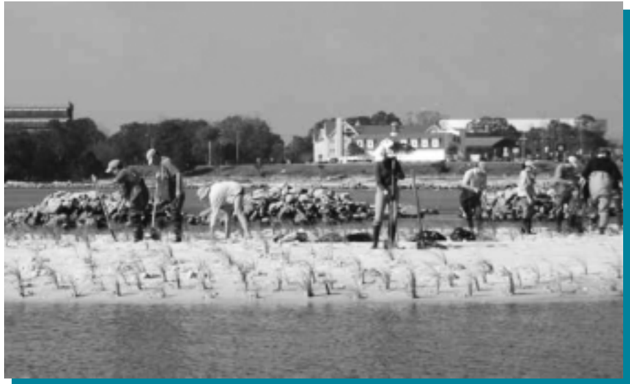
In the final stages of the Pensacola Bay, Florida GreenShores Project, volunteers plant saltmarsh grass behind the newly created oyster reef/breakwater.
