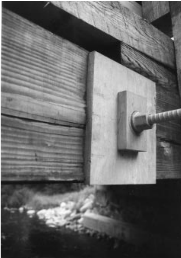
Figure 25—A check in an exterior lamination noted during condition assessment.
