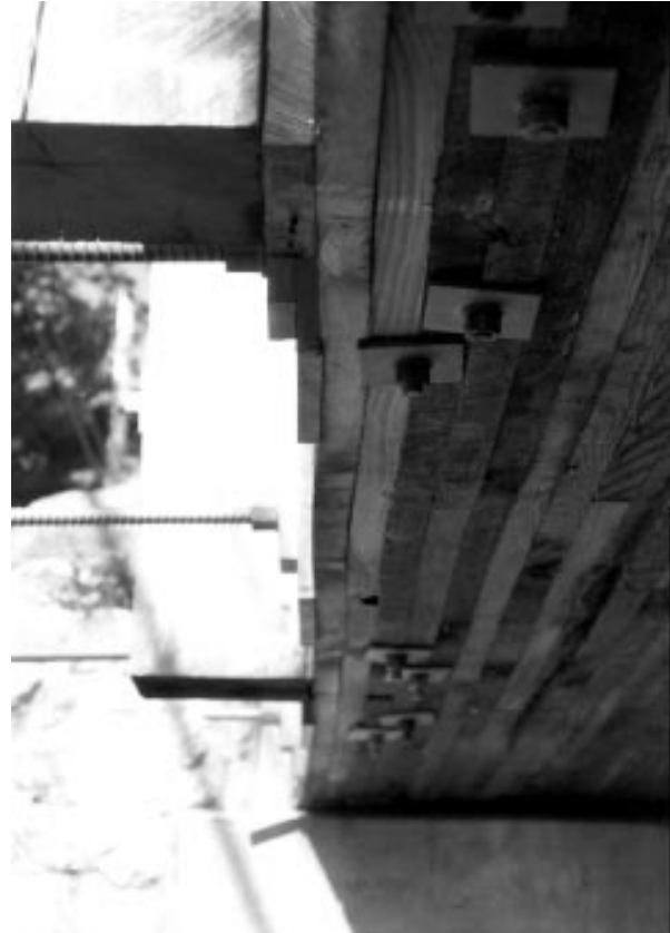
Figure 26—Distorted exterior lumber lamination noted during condition assessment at the time of load test 2.
