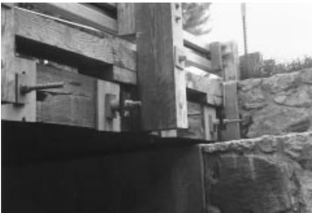
Figure 8—Load cells positioned on stressing bars to monitor bar force.
