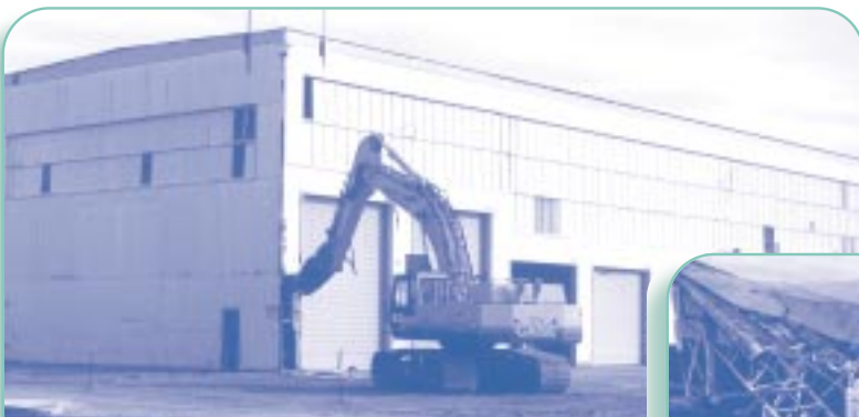
Demolition and remediation of the Central Facilities Area Big Shop: before, during and after
