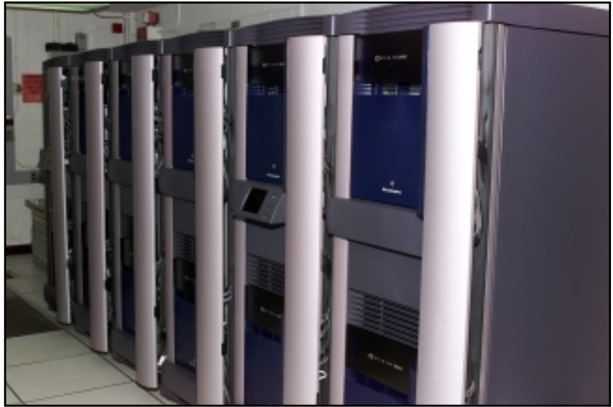
Parallel High Performance Computer Graphics Facility
