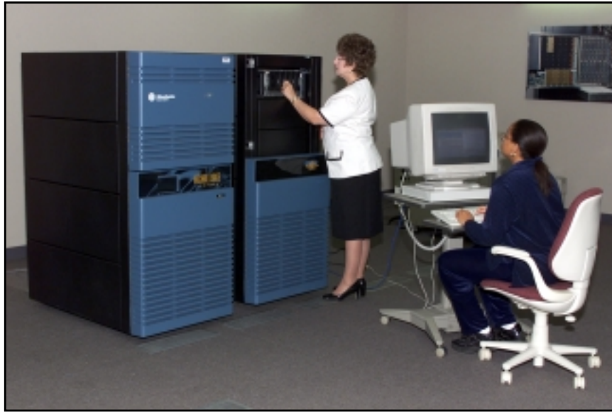
Secure Supercomputing Facility
