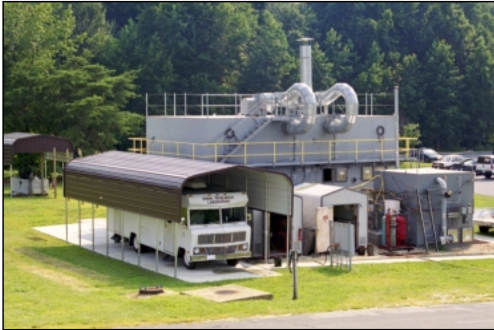
Large-Scale Fire Research Test Bed Facility
