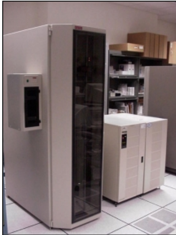
Tape library of the Bergen Data Center
