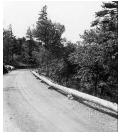
Little is left of the Fitch Overlook due to severe structural failure. Today, Jersey barriers have replaced the historic furnishings, which separate the parkway from the overlook, 2002. Courtesy DCR/Vollmer Team.
