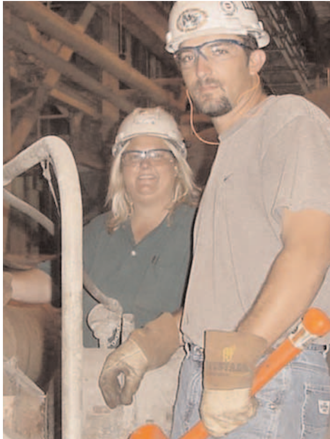
Widows Creek Fossil Plant’s Felicia Blackwell and Matt McLaughlin work on the Unit 7 scrubber absorber pump. They are among 47 graduates of the Fossil Power Group Multi-Skilling Program for new hires.
