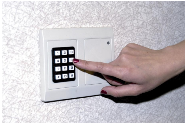
Keypad entry system.
