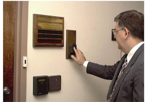
Fingerprint scan used for physical access control.
