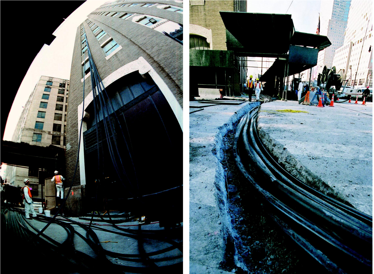
Figure 9: Verizon Used Temporary Cabling Solutions at 140 West Street
