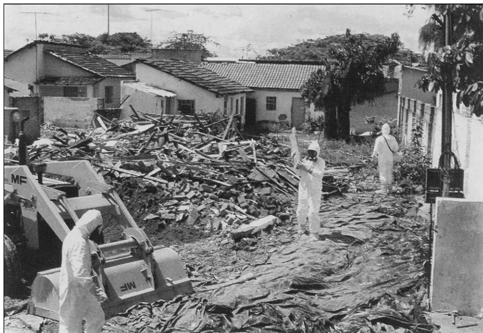
Figure 8: Contaminated Radioactive Debris from Demolished Residences in Goiania
