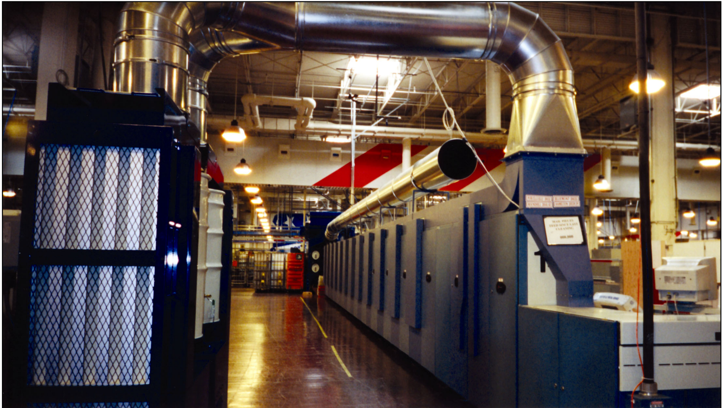
Figure 7: DBCS Torit Air Filtration System
