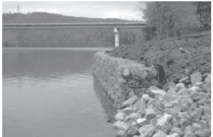
Gabions and Rock Riprap
