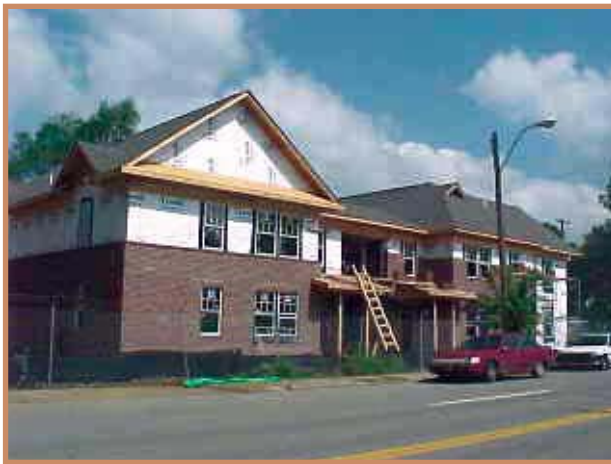
The Memphis Multibank CDC's work in the Greenlaw neighborhood is spurring other redevelopment activities, such as the construction of these new apartment buildings.
