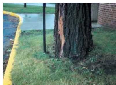
Figure 3.85. Recent construction on three sides of this tree reduces anchoring ability of roots.
