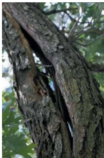
Figure 5.3. Remove the entire branch back to its junction for large branches that are cracked.
