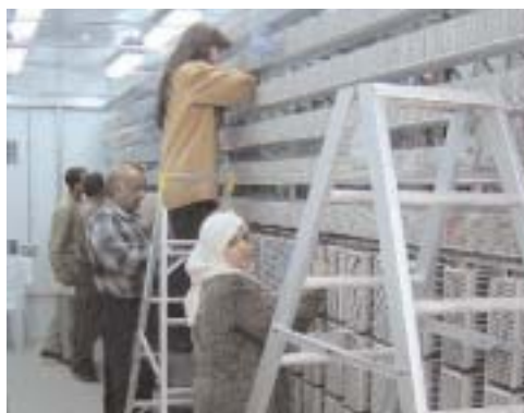
Iraqi Telephone and Postal Company workers connect subscribers in a Baghdad area telephone exchange.
