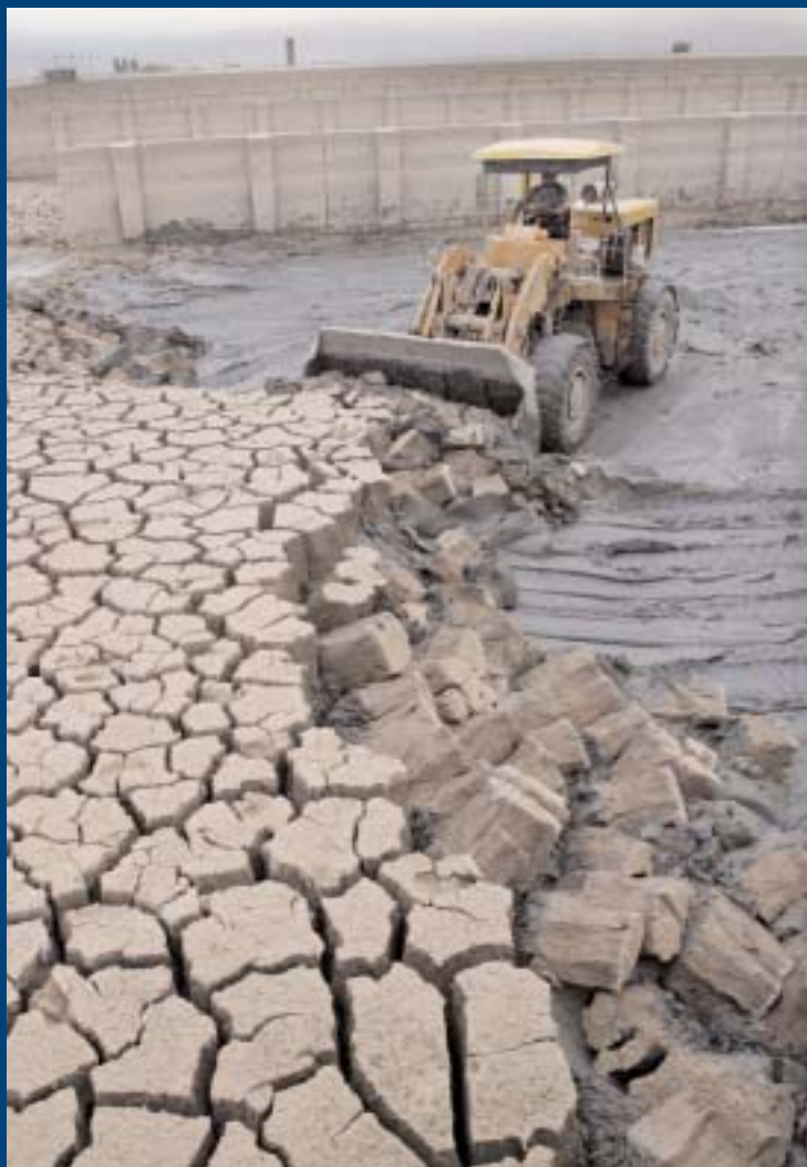
Removing caked silt from Sweet Water Canal reservoirs. The Canal system supplies water to 1.75 million people in Basrah governorate.
