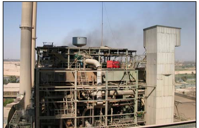
A boiler unit at Baghdad's Doura Thermal Power plant. Photo: USAID
