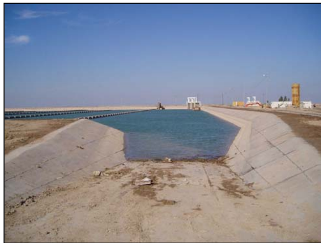
The newly restored west settling-reservoir of the Sweet Water Canal. Photo: USAID
