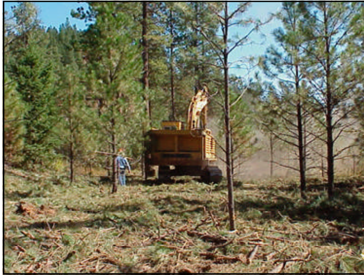
A grinding machine thinning and reducing residual slash at the same time.
