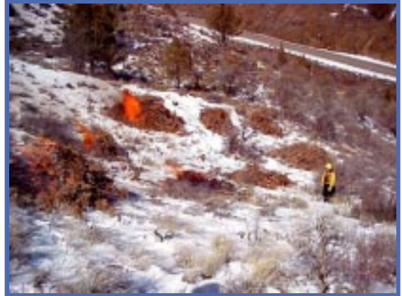
Eight piles of trimmed brush are visible in this photo, an indication of the amount of overgrowth found on the site at the start of the project.
