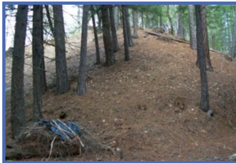
Completed section of fuel break with piles of removed vegetation ready to be burned.
