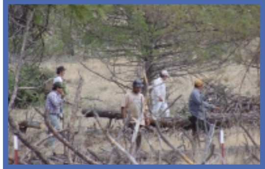
Contract crew performing chainsaw thinning and hand piling on BLM land at Bly.
