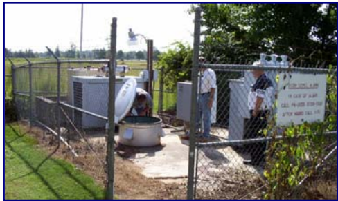
Original lift station
