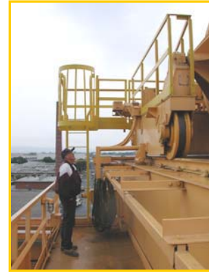
Safety guardrails installed on bridge crane prevent falls
