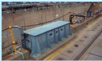
Post and chain system was replaced by guardrails to improve fall protection.
