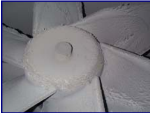
Over 25 pounds of paint residue were removed from fan blades and ductwork
