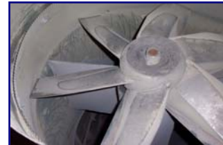
Fan blades after cleaning
