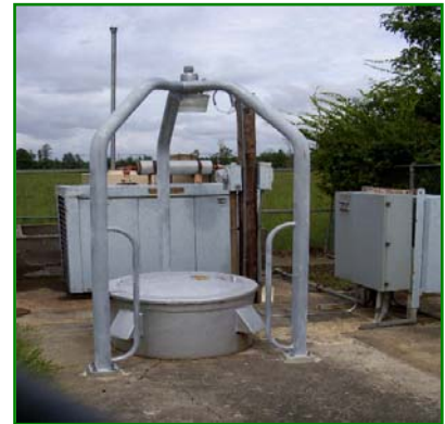
New lift station rescue system anchor
