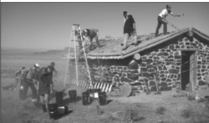
Volunteers repairing the roof of a Pony Express Station near West Desert, Utah.
