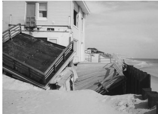
A deck collapsing as a result of coastal erosion.
