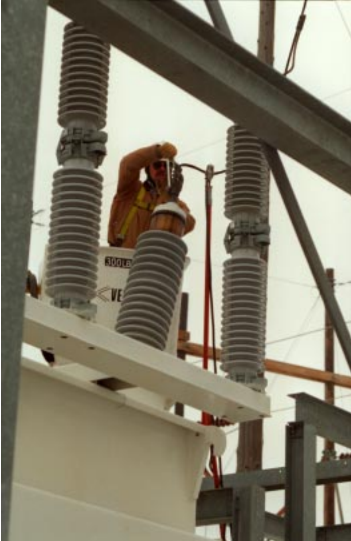
INEEL linemen use every precaution in working on high-voltage lines, substations and transformers. The INEEL workforce includes numerous electricians, welders, carpenters, pipefitters, mechanics, equipment operators, and other craftsmen.
