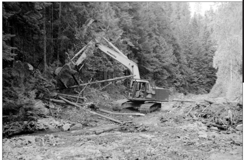
Riparian area stream restoration from mining damage near Pinecreek (Coeur D'Alene Field Office, Upper Columbia - Salmon Clearwater BLM District).
