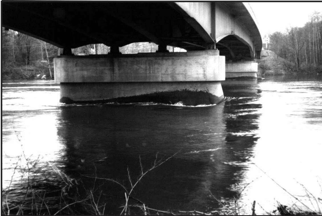
Figure 3. River flow near bridge piers on Androscoggin River at Bethel, Maine, April 1, 1998.
