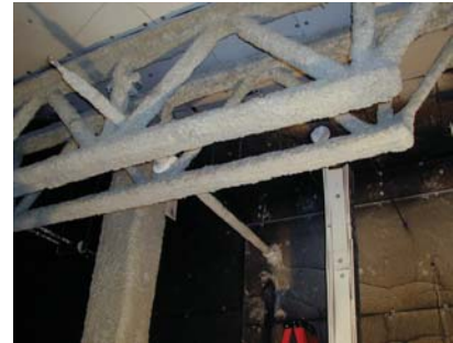
Insulated steel trusses, steel rod, and steel column inside the NIST Large-scale Fire Laboratory
