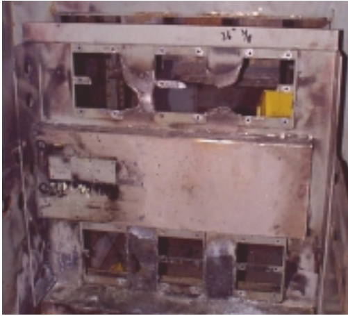
Remnants of exploded switchgear
