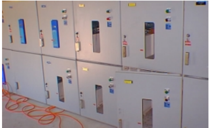
Views of one of the aging transformers
