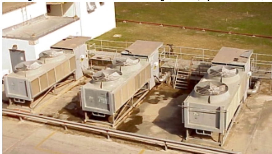
Existing HVAC chiller units (being replaced under currently funded contract) are representative of the age of the majority of the facility's HVAC systems.
