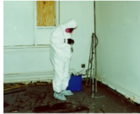
Asbestos Analyst and Safety Specialist, Thorgrimur Arnason, collects samples for clearance following asbestos ripout operation.
