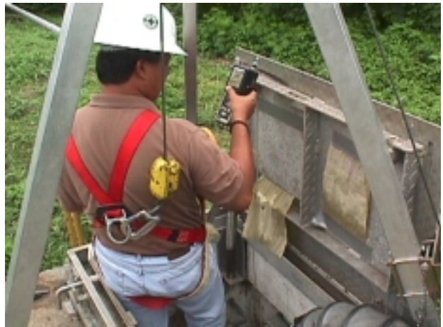
Wearing fall arresting gear to enter and work in a confined space.
