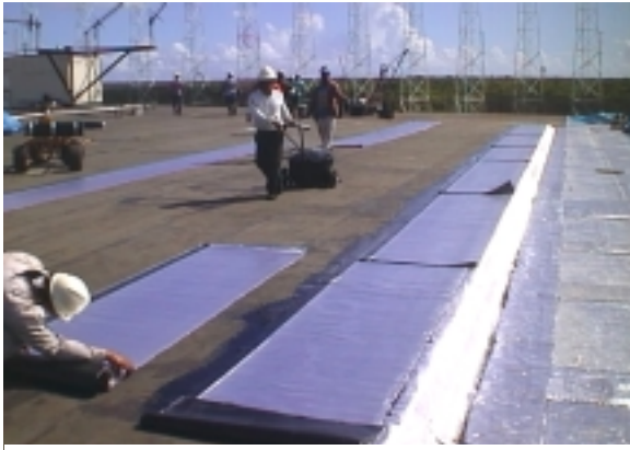
A rooftop perimeter wall is installed to avoid the need for individual fall arrest systems.
