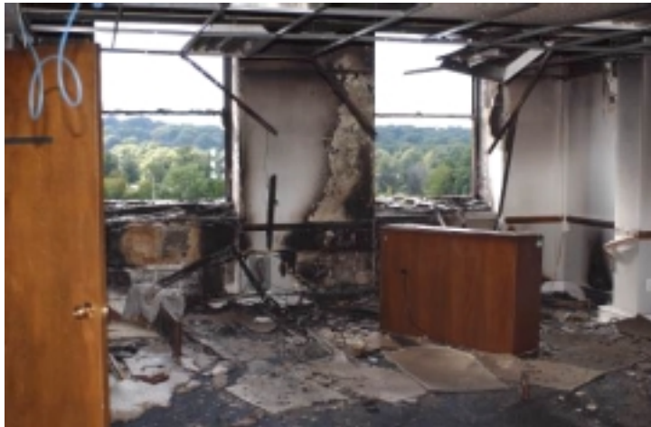
Pentagon office damaged in September 11, 2001 terrorist attack
