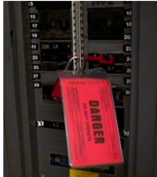
Danger tag warns against energizing electrical power panel.
