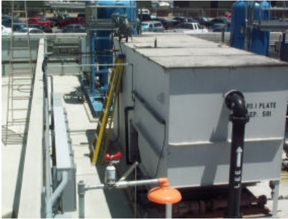
Fall Protection & Prevention Training includes examples of unsafe designs like this Oil Water Separator System accessed only by steep ladders
