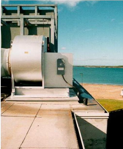
Rooftop ventilation system was designed without fall protection systems for safe access
