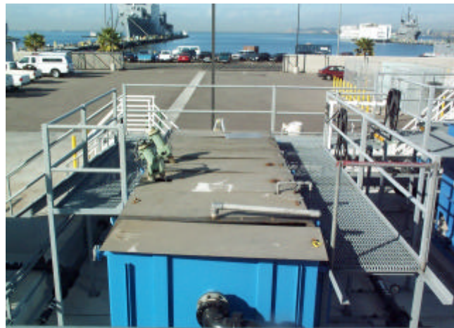
Costly redesign to provide catwalk platforms around Oil Water Separator Systems allows operators and mechanics safe access to equipment
