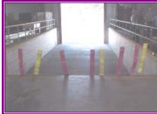
Inclined ramp allows mail trucks to line up evenly with loading dock
