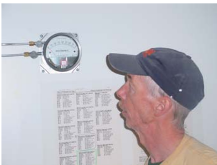
Air pressure gauge tells painter when air filters need changing.
