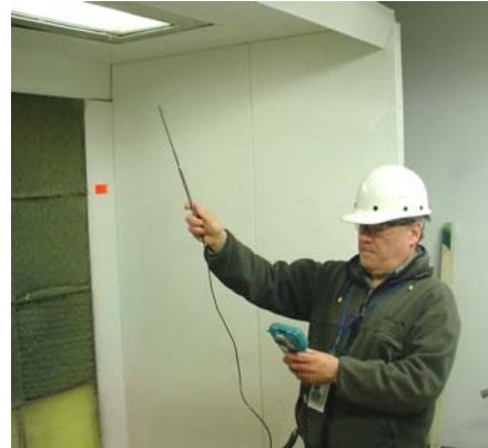
Airflow measurements indicate new spray paint booth exhaust system removes harmful paint
