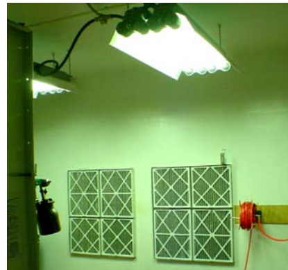
New fluorescent lights, electric outlets, and ventilation fans improve paint room and booth working conditions.
