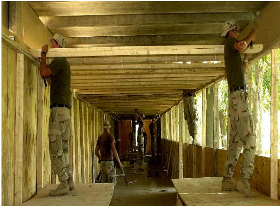
Naval Mobile Construction Battalion Seven Seabees construct an administrative building in Ad Diwaniyah, Iraq.
