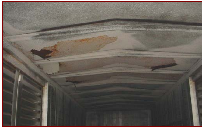
Damaged ceiling tiles in railcar in need of repair
