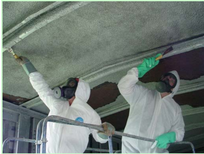
PWC clean up team members, wearing protective clothing, scrape railcar ceiling tiles in preparation for painting
