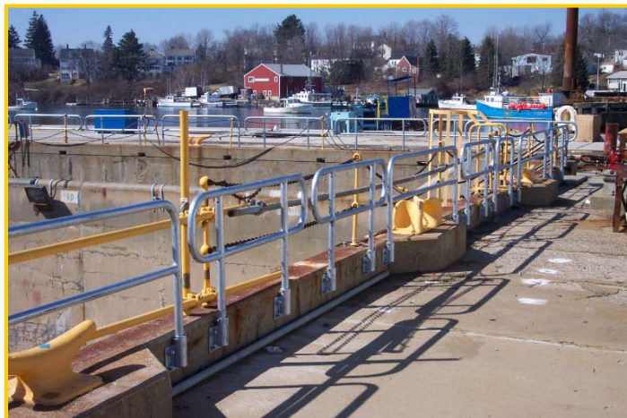
Guardrails, with toprails, midrails, toeboards, and posts, around the perimeter of PNS dry-dock
