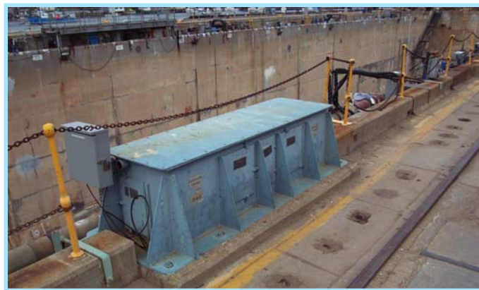
The post and chain system, shown above, was replaced by guardrails that improve protection from falling into the dry dock.
