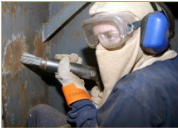
A sailor uses a needle gun to remove layers of paint during USS John F. Kennedy's ESRA period.
