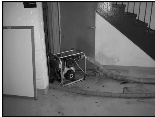
Discharge pump helped to remove floodwater from first floor of NRC Baltimore
